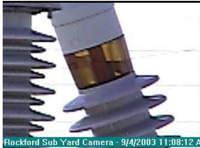
Figure 2. The oil level is clearly apparent in this 69,000 volt transformer bushing.
