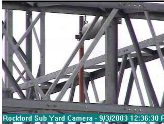
Figure 7. Intact high-side fuse indicates the cause of a low-voltage problem lies upline.
