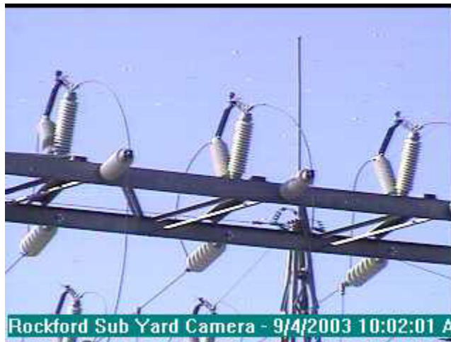
Figure 4. Visual confirmation of closed switch position.
