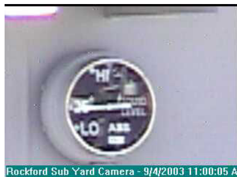
Figure 3. Liquid level gauge viewed from approximately 300 feet.
